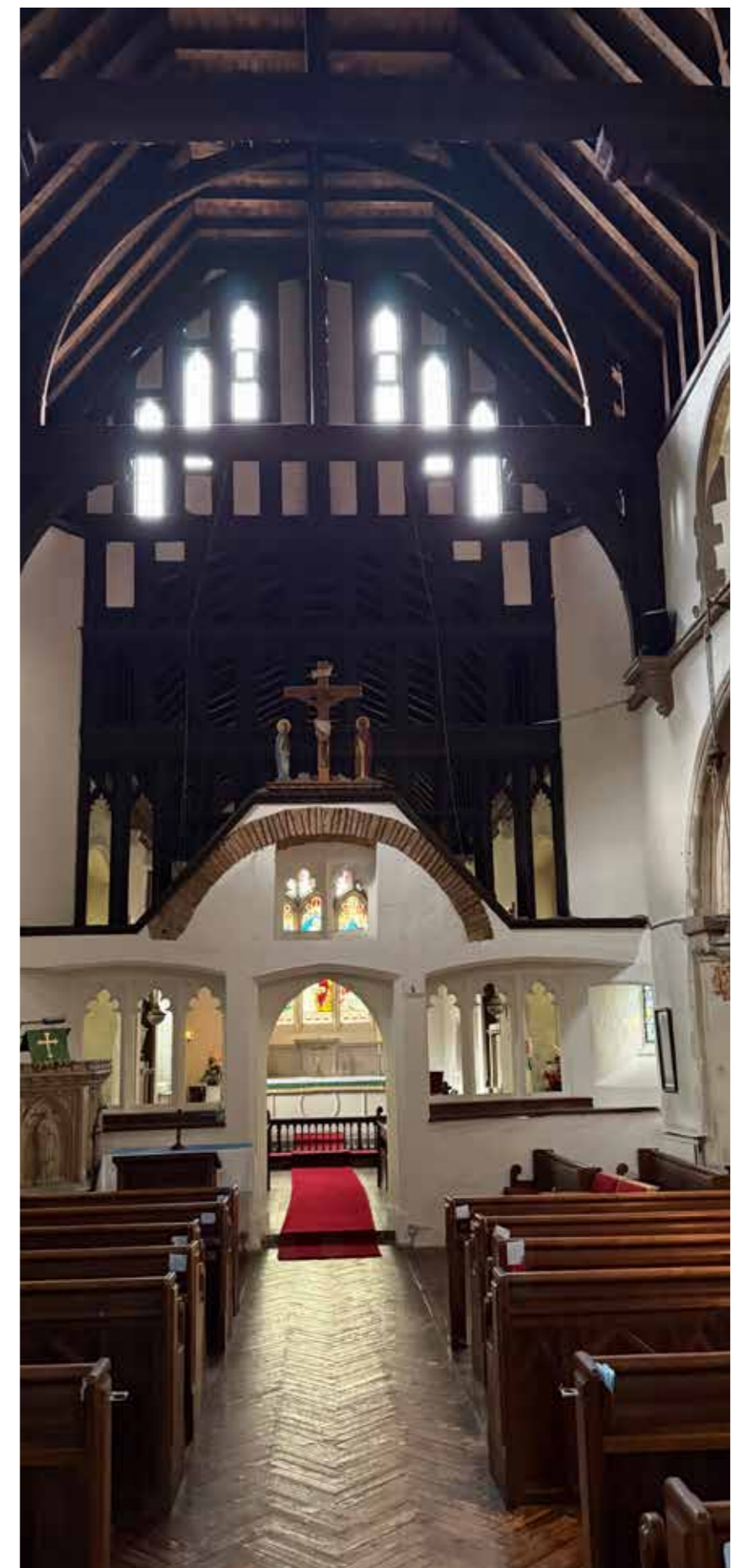
Lattice screen over by William White designed to disperse the load of the raised nave roof.
